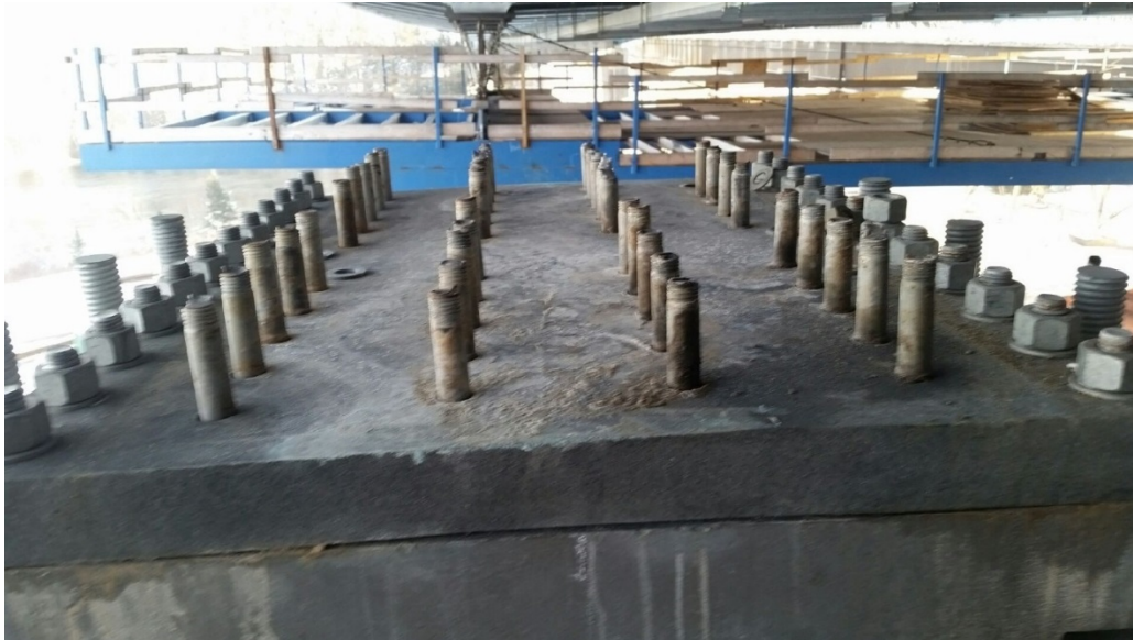
Figure 1-2: Fractured bolts (ASTM A490 bolt - connecting shoe plate to girder flange) and deformed shoe plate at north-west bearing. Note four lines of failed flange connection bolts.
