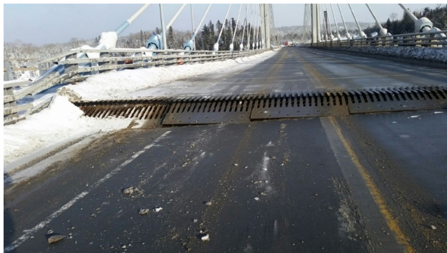
Figure 1-1: Nipigon River Bridge, 600mm uplift of north bridge edge at west abutment, January 10 th , 2016
