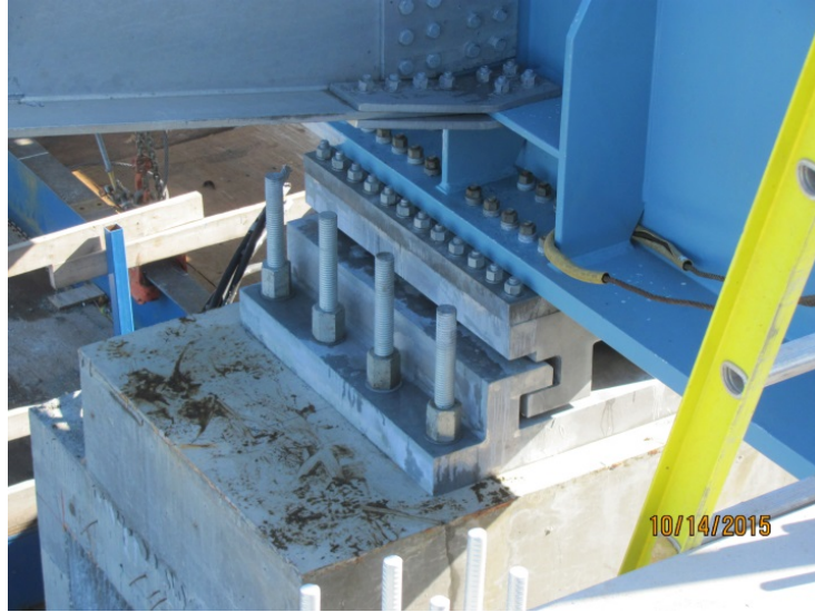
Figure 1-4: Centre-west bearing in place. Bevelled shoe plate is seen between girder flange and bearing sole plate.
