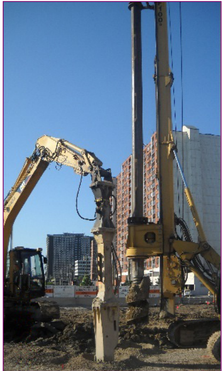
Figure 1: Rammed aggregate piers are placed within the foundation footprint of the new Canadian Border Services Agency Building in Windsor.
